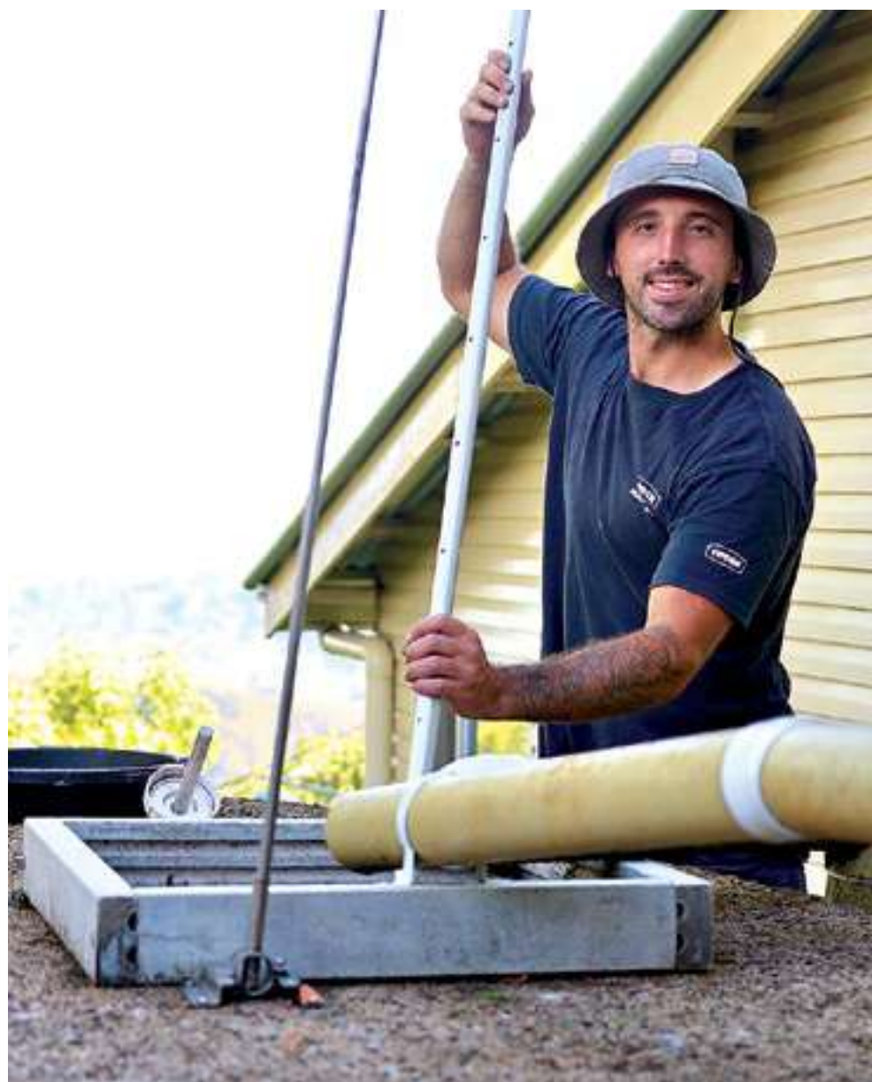
Ryan Davies is a plumber by trade so he can also check and make sure your pipes and taps are in good working order.
