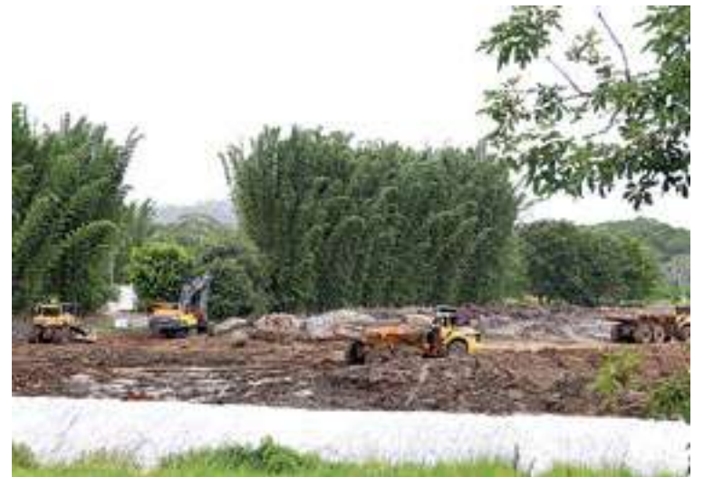
Extensive earthworks are being carried out on the site, much to the annoyance of some locals..
