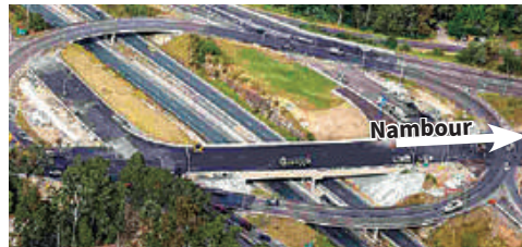
The bridge section to be demolished is the arc closest to the bottom of photo.
