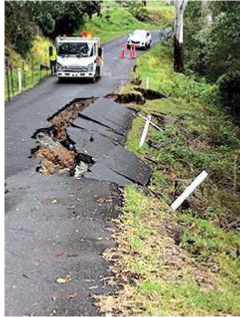
Major damage to Hovard Road at Bald Knob.
