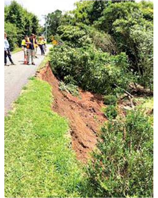
Landslip: Policeman Spur Road, Booroobin.
