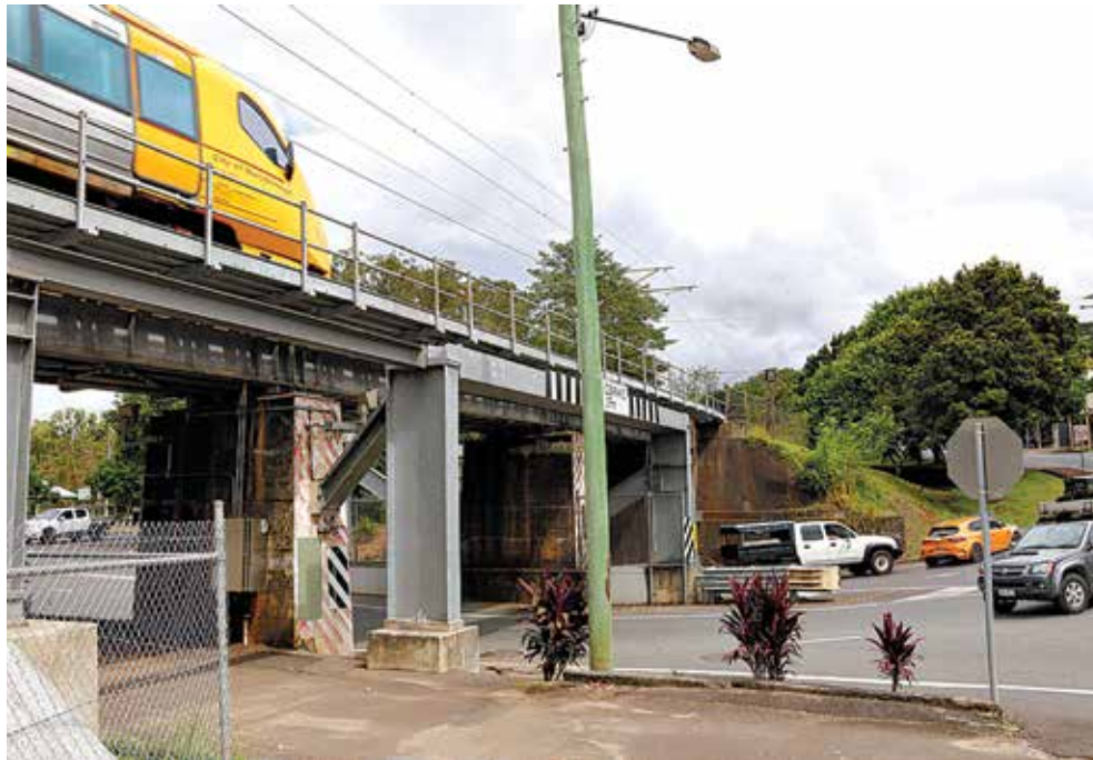
The rail bridge intersection in Palmwoods. It needs major work but who's going to pay?
