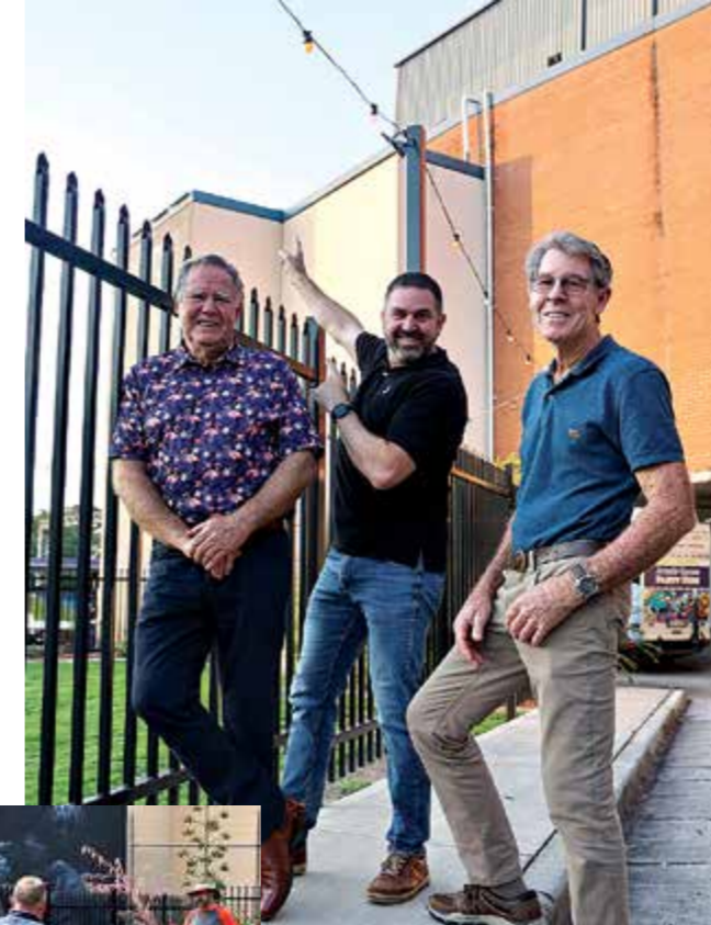
Above from left: Greg Rogerson, Darren Shepherd and Peter Clark installed the lighting which will illuminate night time functions at the terminus in Mill Street. Left: Ten four metre high stainless steel poles crowned with LED floodlights now shine down on backyard of the terminus.
